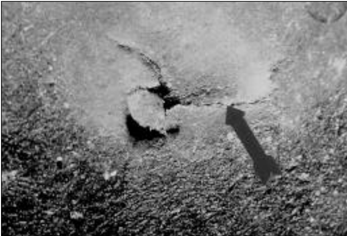
Photo A7. Close-up on bottom side of Tab G-3 at area depicted in Photo A6.
