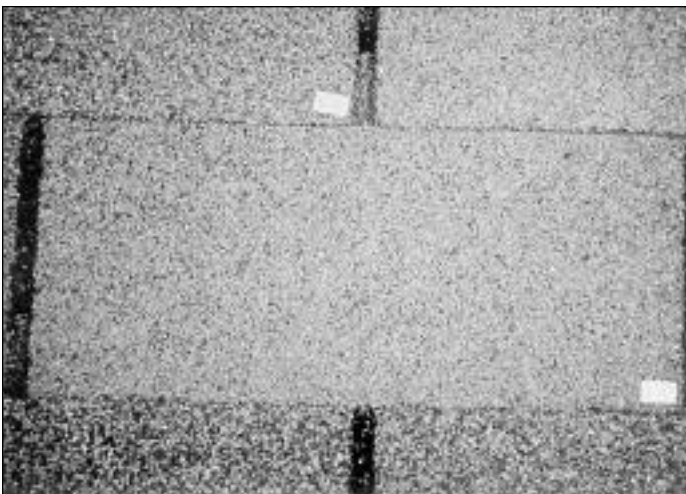
Photo C2. Close-up of Tab C-5 before impacting at 10 years 5 months weathering exposure.
